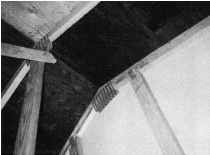
FIGURE 11.26 Example of fully serviceable untreated plywood roof sheathing (top left) adjacent to thermally degraded FR-treated plywood sheathing (center) used next to a gypsum-sheathed 60-minute-rated fire wall (lower right).
