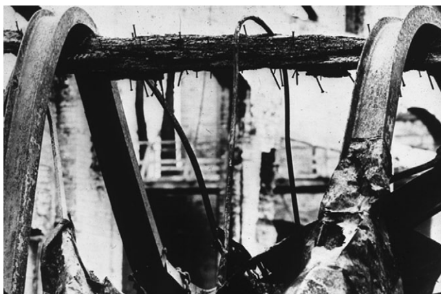
FIGURE 6.7 Wood beam survives fire in casein plant in Frankfort, NY.
